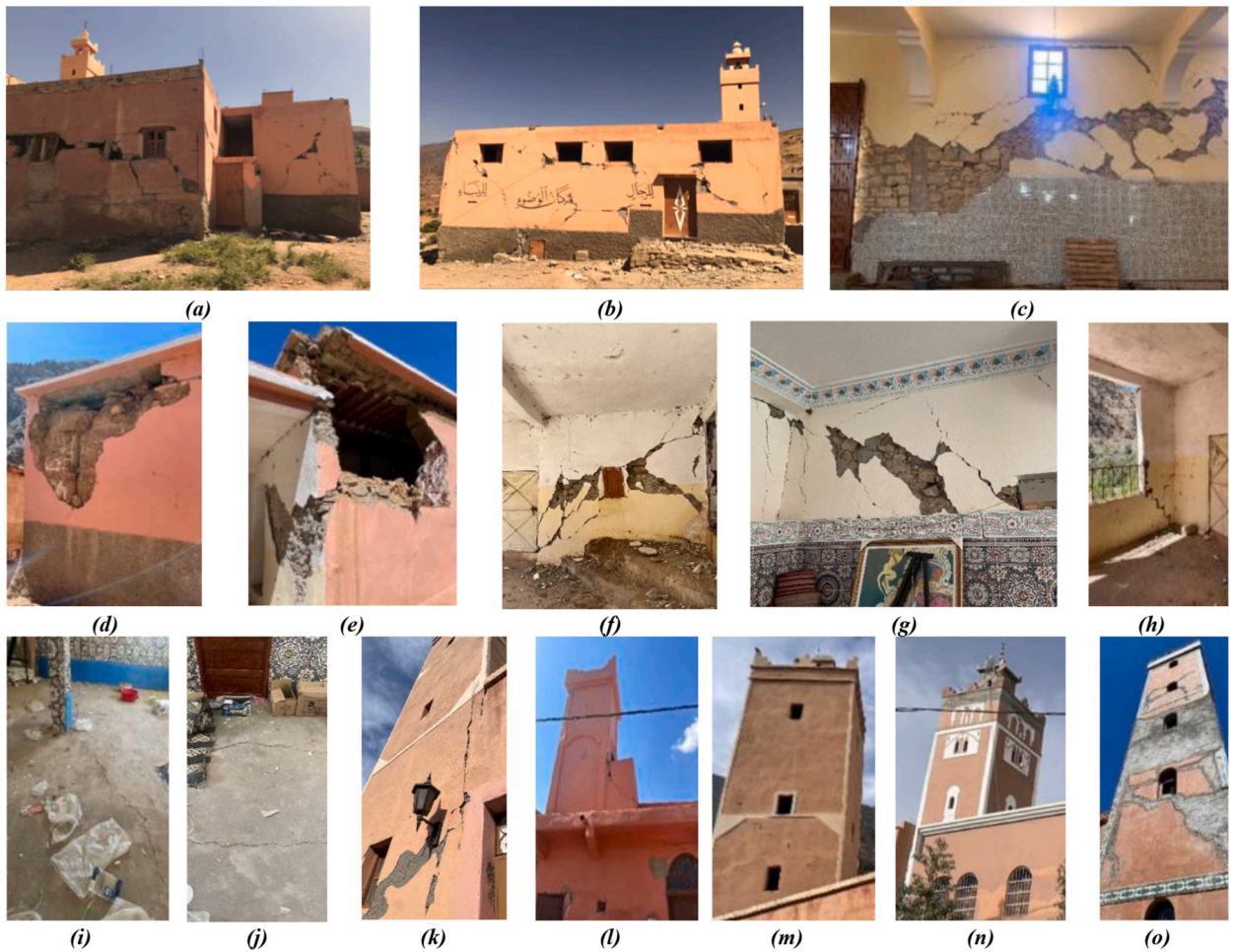
Fig. 30. CM mosques with CMU infill panels showing: (a–b) severe diagonal and X-shaped widespread shear cracking and partial collapse of infill panels; CM mosques with SM infill panels showing: (c) diagonal and horizontal infill separation cracks along with plaster detachment, indicating poor frame–infill interaction; URM mosques with RE and SM showing: (d–e) partial collapse of external walls, (f–g) diagonal shear cracking of internal walls, (h) opening corner cracks, (i–j) floor cracks; Minarets showing: (k) pounding damage; (l) partial collapse of unreinforced upper parapets; (m) diagonal shear cracking of infill panels; (n–o) repair interventions.
