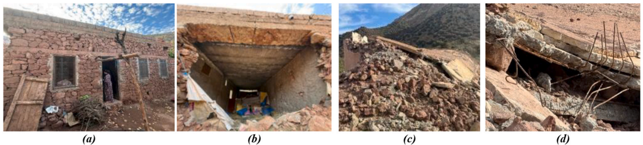
Fig. 24. (a) SM building with RC beams at lintel and roof levels; (b) out-of-plane wall dislodgement from the RC beam; (c) RC roof collapse; (d) failure of a lightly reinforced RC slab.
