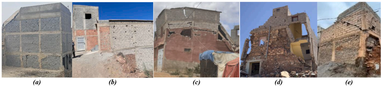
Fig. 26. Permanent housing: (a) without finishes, (b) with partial finishes, (c–e) observed failures of hybrid buildings.
