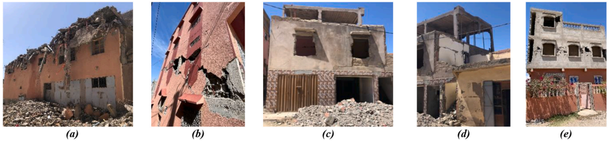
Fig. 27. Reinforced concrete (RC) buildings in settlements close to the epicentre: (a) failure of upper storey; (b) shear cracking in infill walls; (c–e) dislodgement and loss of infill panels.
