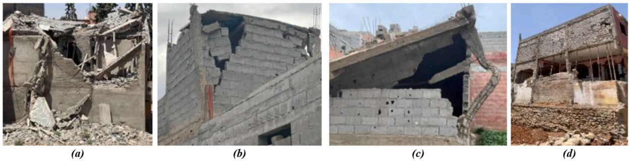
Fig. 15. Confined Masonry (CM) buildings showing roof failure driven by: (a–b) overturning of panels; and failures at beam–wall (c) and column–wall interfaces. CM building showing (d) panel dislodgement and material loss in columns with exposed reinforcement.
