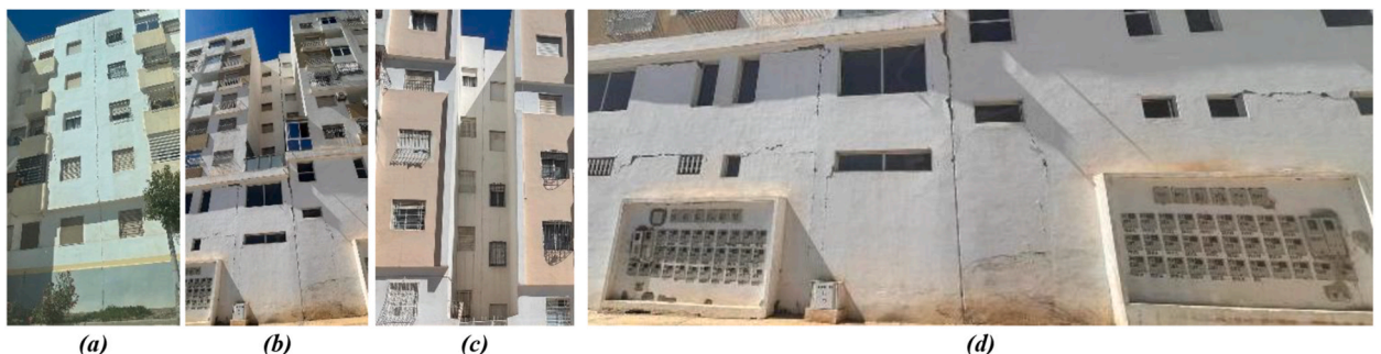
Fig. 28. Reinforced concrete (RC) buildings in Agadir: (a–c) Cracking observed at seismic joints; (d) Light damage to non-structural elements.
