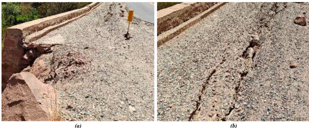
Fig. 9. Tension cracks and damage to small retaining structures along the R202/N7.
