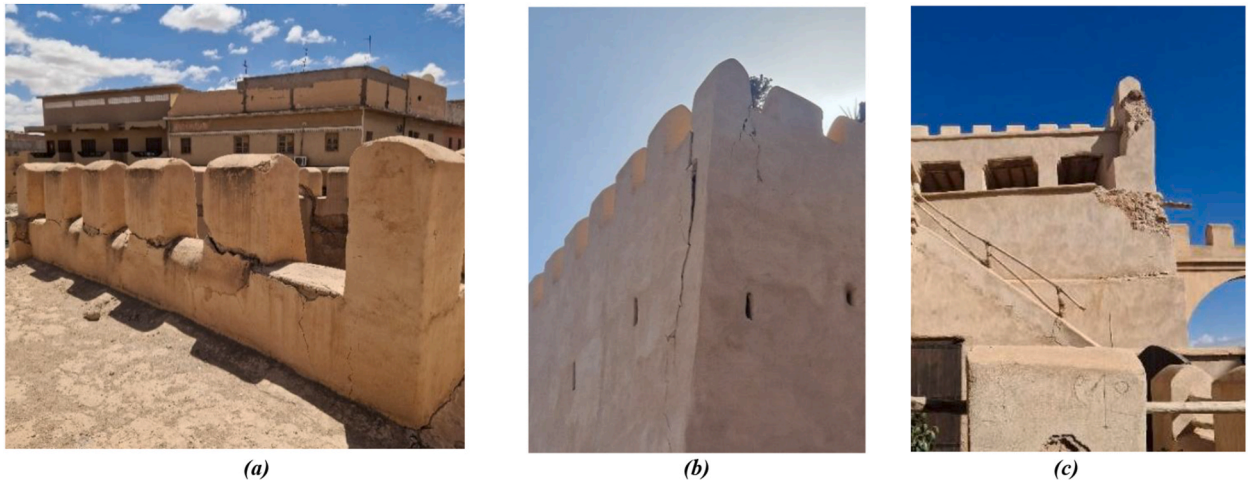
Fig. 41. Babs of Taroudant city wall: (a) out-of-plane cracks at the base of merlons at Bab Targhount; (b) vertical corner cracks at Bab Ouled Bonouna; (c) partial collapse at the top of the wall at Bab Ouled Bonouna.
