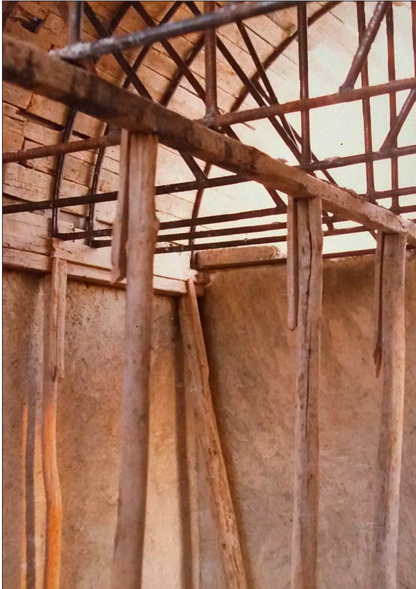
Figure 15: Formwork made by a builder at Milihouse for his own family's vaulted house. The formwork is inspired by that used in the Milihouse project. Source: Mousally (1988: 100).
