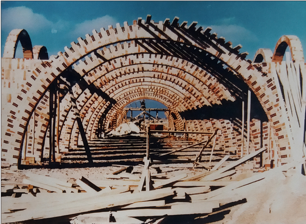
Figure 3: This vaulted project in Syria, built between 1987 and 1988, is the Al-Khaldiya Farm, designed by Abd Alfattah Iyas, Andre Mashaqa, and Amer Mousally. The structure's diaphragm vault is of brick arches with barrel vaults. Source: Mousally (1988: 92).
