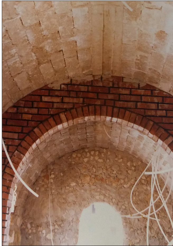
Figure 14: Interior of a vaulted space in Al-Sharqyat. Construction of first experimental houses in Al-Sharqyat using local materials, and vaults for the second floor. Source: Mousally (1988: 100).
