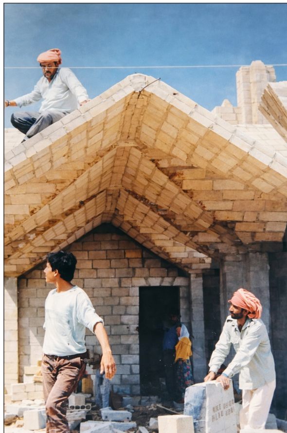
Figure 1: A vaulted house in Syria, built between 1987 and 1988, designed by Rabie Dahman. The house’s roof is folded and made of cement blocks, reducing the need for steel reinforcement. Source: Mousally (1988: 78).
